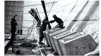
John Day Lock anchor caps and exposed anchor tendons
