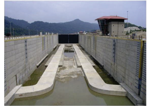
In-chamber longitudinal culvert system; Marmet Lock, Kanawha River
