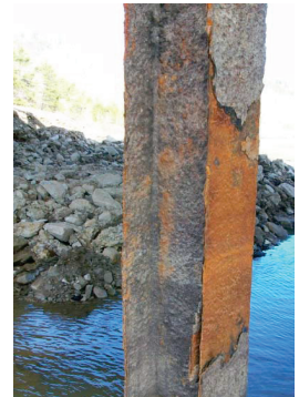
Corroded Steel H-Pile on East Fork Bridge
