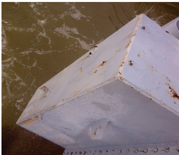
Figure 5: This trunnion anchor rod cover box indicates multiple rods have failed in the anchorage.
