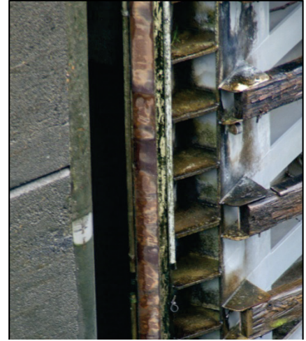
Corroded steel miter blocks
