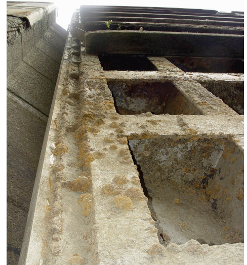
Corrosion on miter gate at Selden Lock, AL
