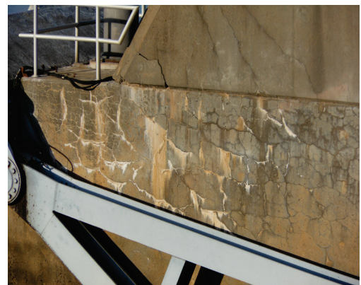
Figure 6: Severe alkali-aggregate reaction damage at David Terry Lock and Dam, constructed in 1968.
