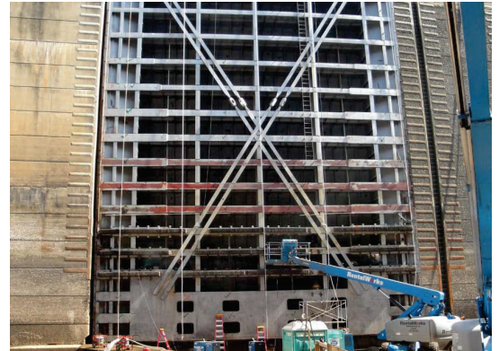
Typical horizontal framed miter gate at Holt Lock
