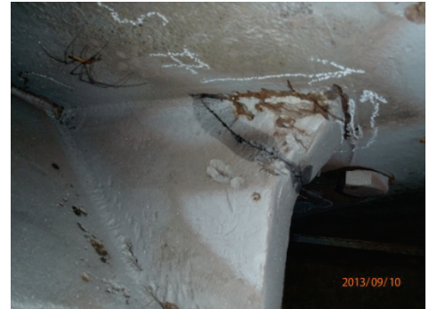
Damaged Pintle Socket, Aberdeen L&D
