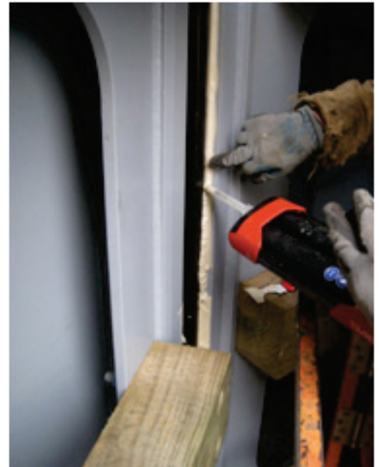
Sealing lock gate quoin block
