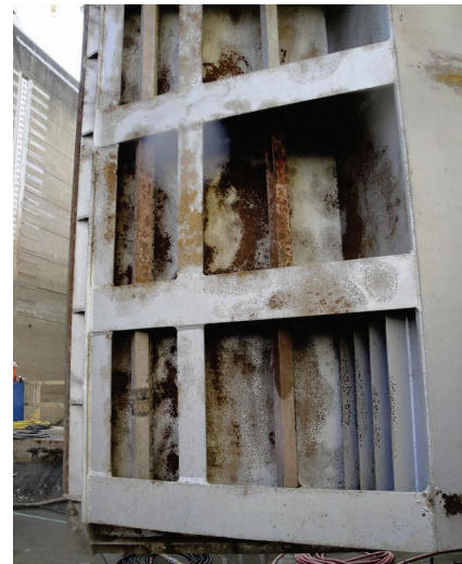
Corrosion on miter gate at Claiborne Lock, AL
