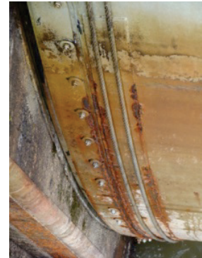
Example of normal breakdown of a coating system on a tainter gate as it ages
