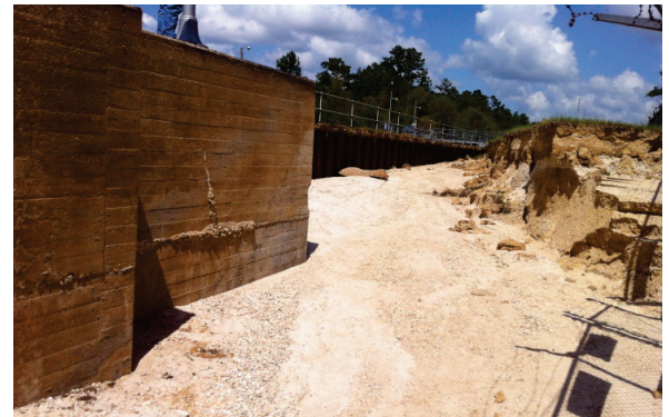
Pearl River Lock, damaged after hurricane surge caused massive erosion during overtopping
