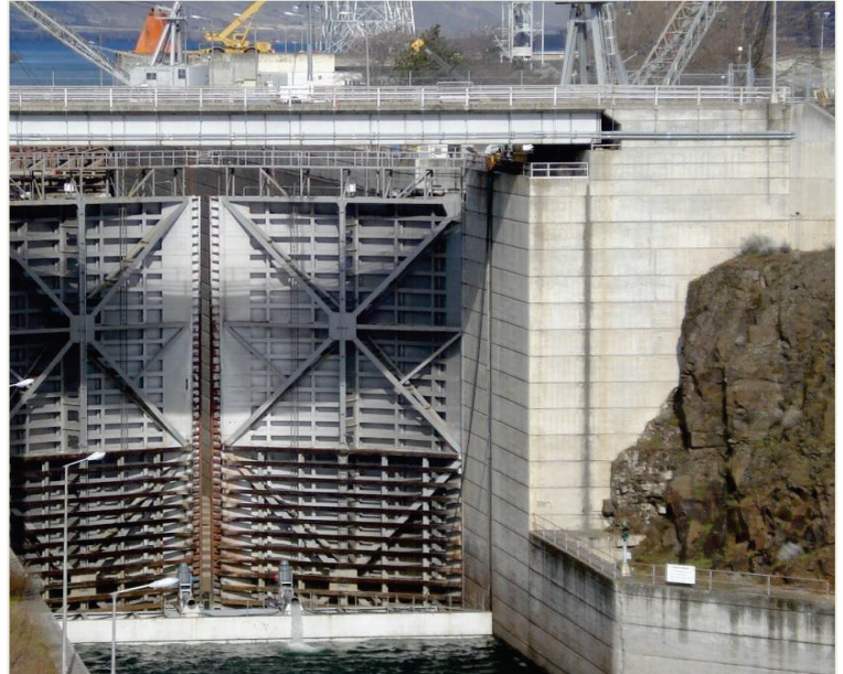
The Dalles downstream miter gates; The Dalles, OR
