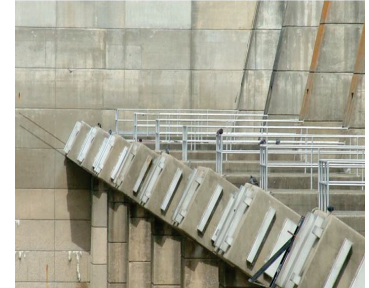
Trunnion rods ejected from pier
