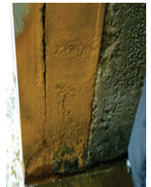
Embedded, Corroded Steel
