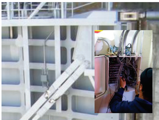
Figure 2: Multiple sensors are installed and wired from the downstream miter gates to a data logger at The Dalles.
