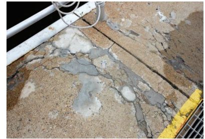
Typical deterioration of horizontal concrete surfaces
