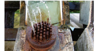
Corroded anchor allowing water flow during lockage
