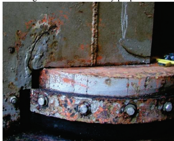
Figure 3: Cracks in a miter gate near the pintle resulting from improper contact between the gate's contact blocks and the quoin blocks.
