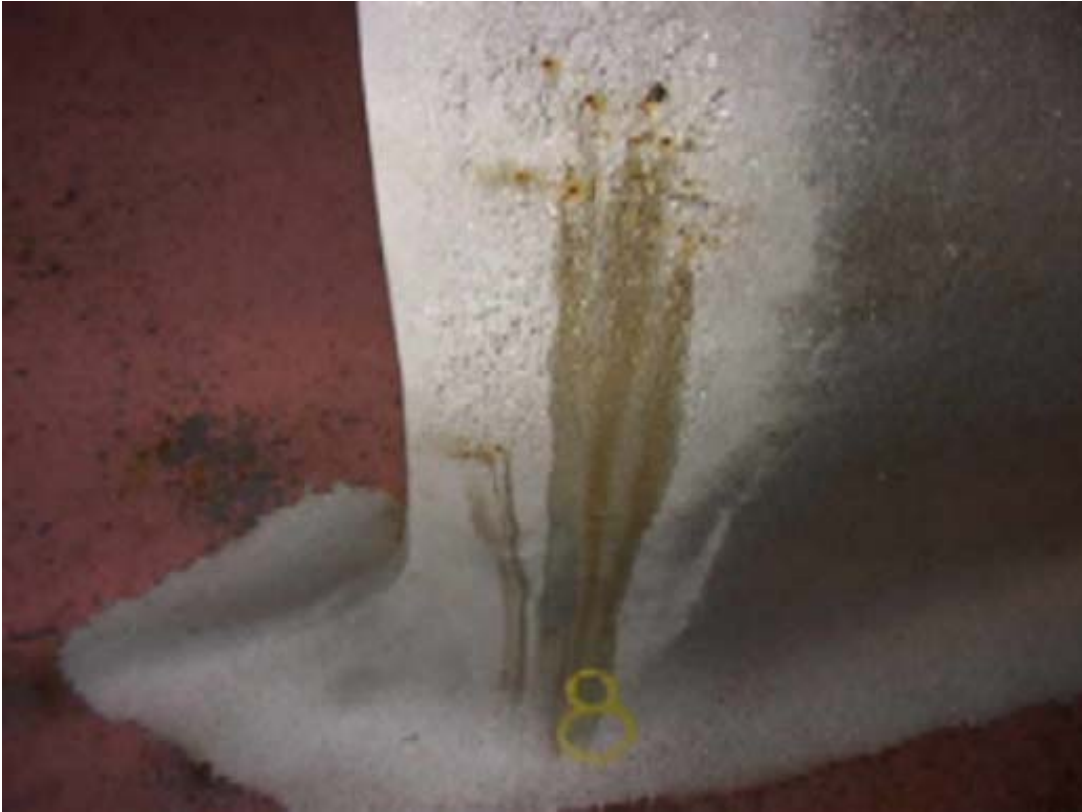
Figure A-1: Stainless Steel – Fair Condition.
