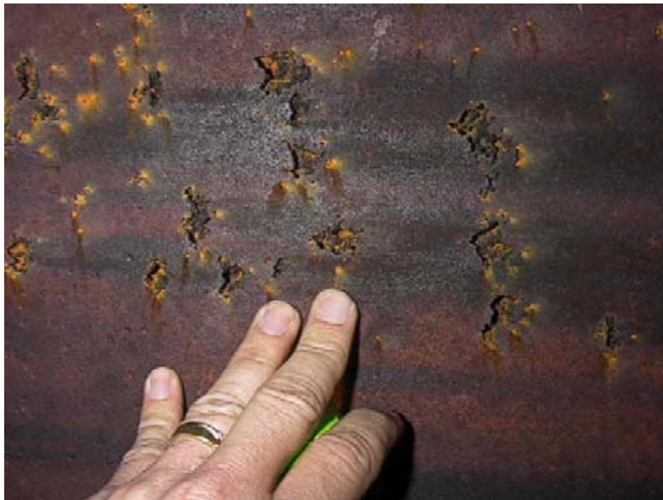
Figure A-3: Carbon Steel – Fair Condition (pitting).
