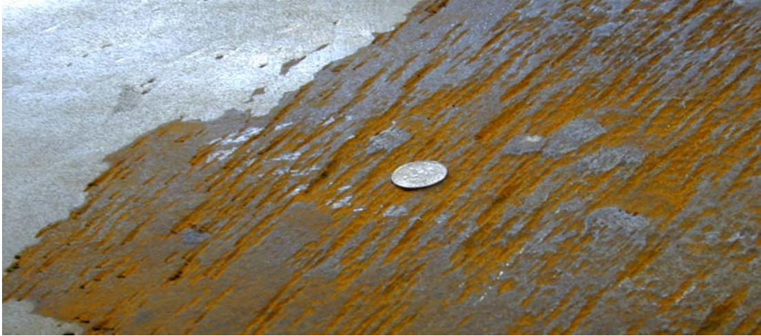
Figure A-5: Carbon Steel – Poor Condition.
