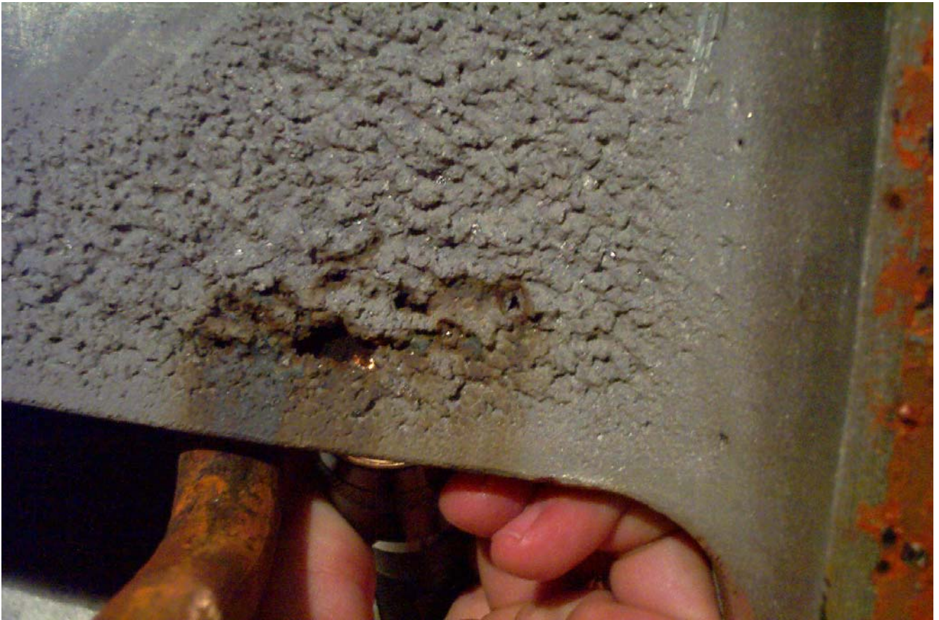
Figure A-7: Carbon Steel – Poor Condition.
