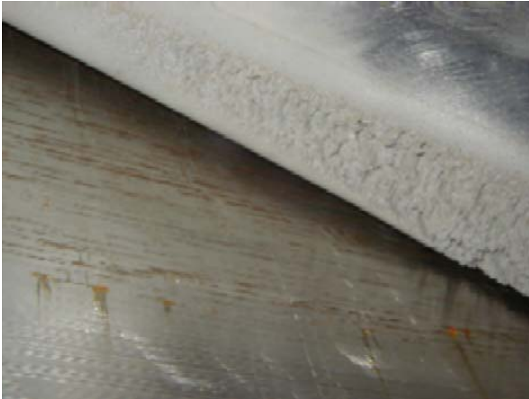
Figure A-2: Stainless Steel – Poor Condition.
