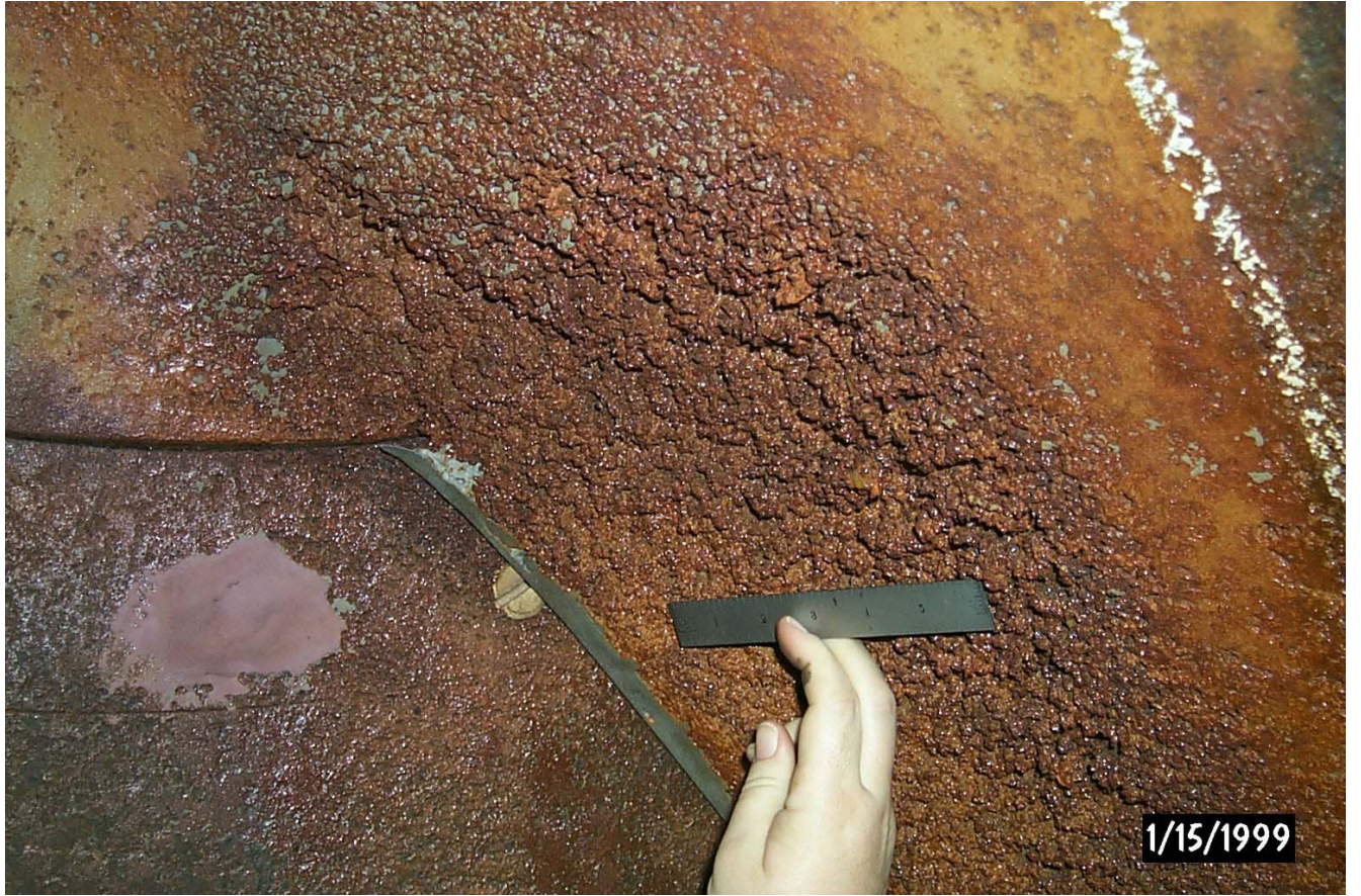
Figure A-4: Carbon Steel – Poor Condition.
