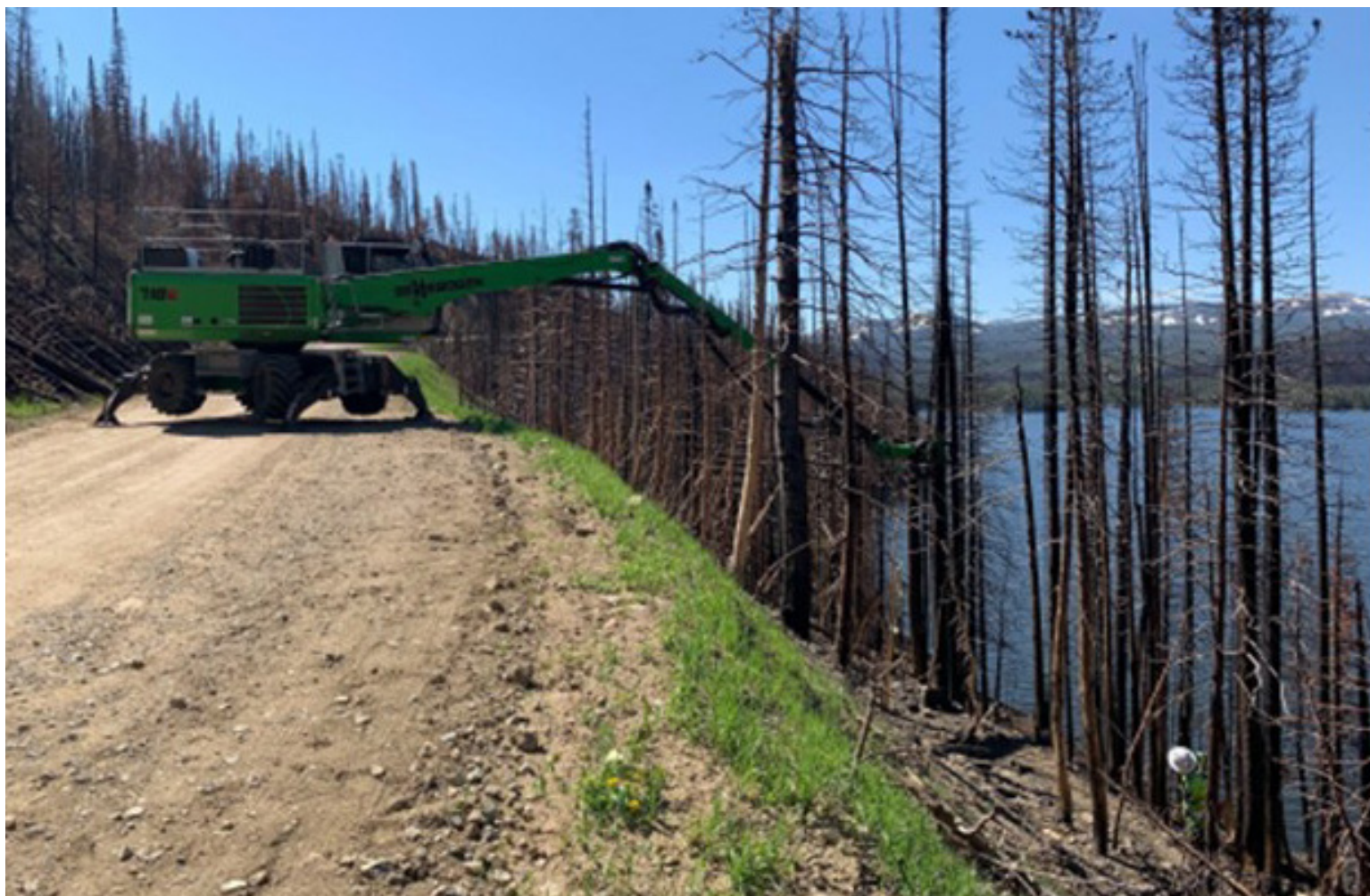
Debris removal / hazard tree removal efforts following the Cameron Peak Fire. Note the water source at the bottom of the steep hill. (Source: K. Parrott Presentation, 18 Oct 2022)
