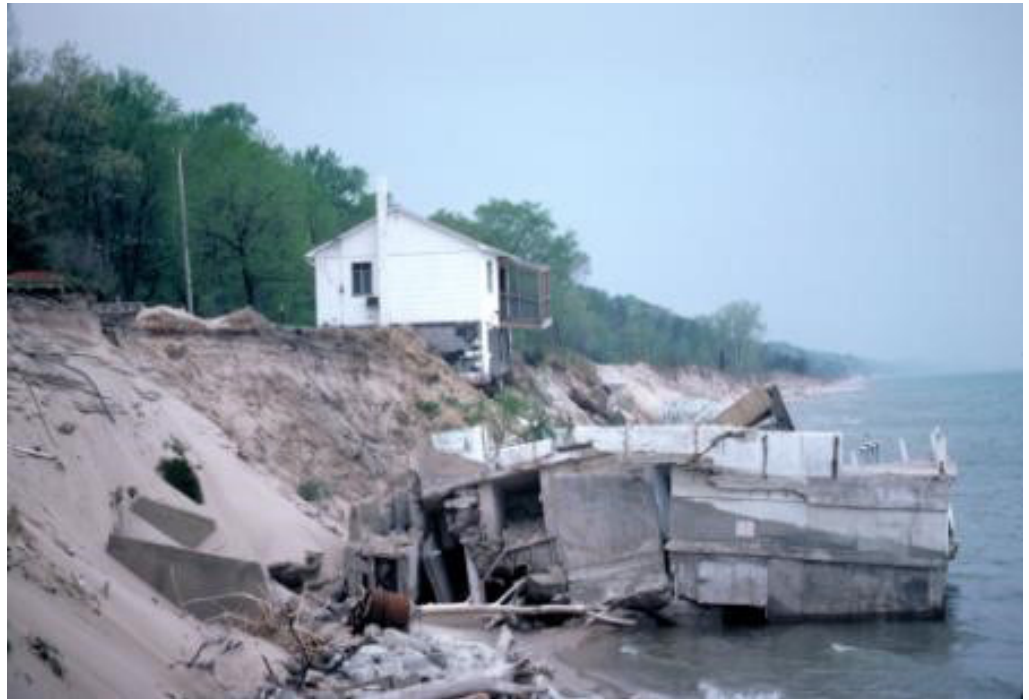
Shoreline erosion in Indiana. (EPA GLNPO)
