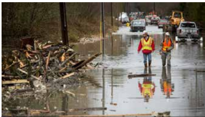
Douglas Weber and COL Bruce Estok evaluating the damage on SR 530 caused by the Oso Landslide
