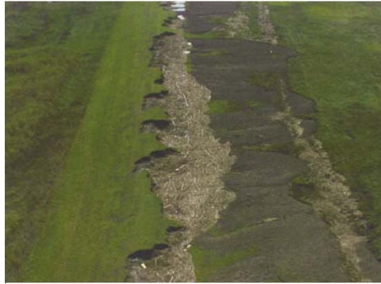
Levee damage caused by Hurricane Katrina (protected side is to right in photo).
